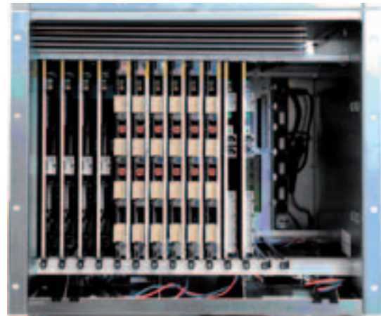
Control and Switching Module
